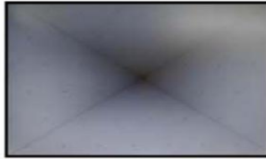
Abnormal Power Section
